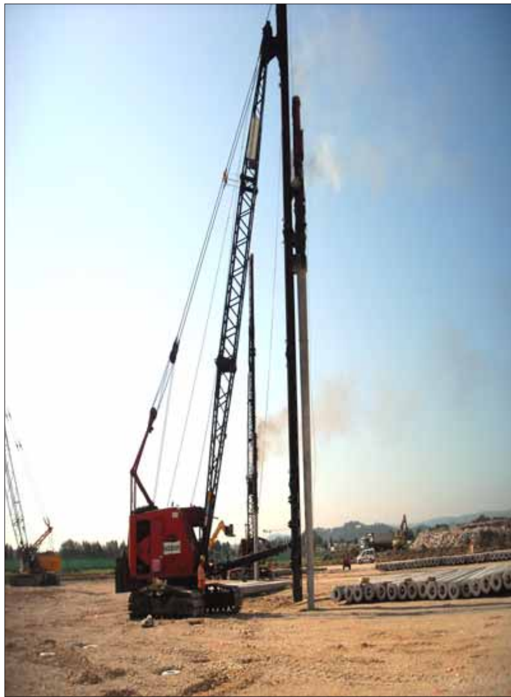
MAKING PROGRESS: Pile driving machines work full speed at Dal Molin for the foundations of the $289 million multiple facilities complex scheduled to be completed in the summer of 2012. SEE PAGE 3 for the Italian language version of the Dal Molin update.
